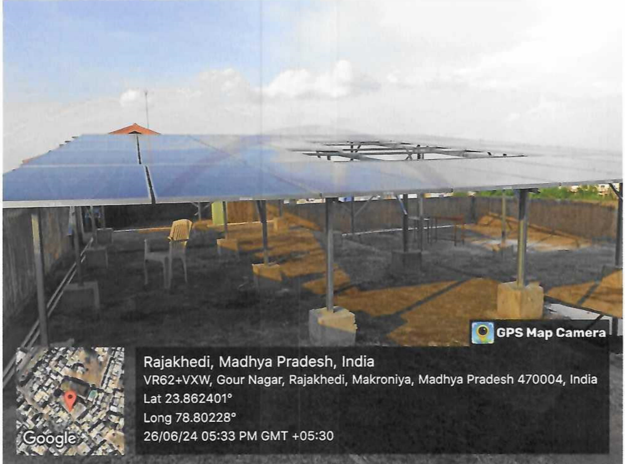
Solar Panel System
