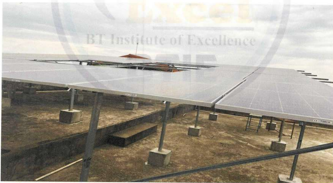
BTIE SOLAR PLANT INSTALLED IN ROOF TOP OF THE BUILDING
