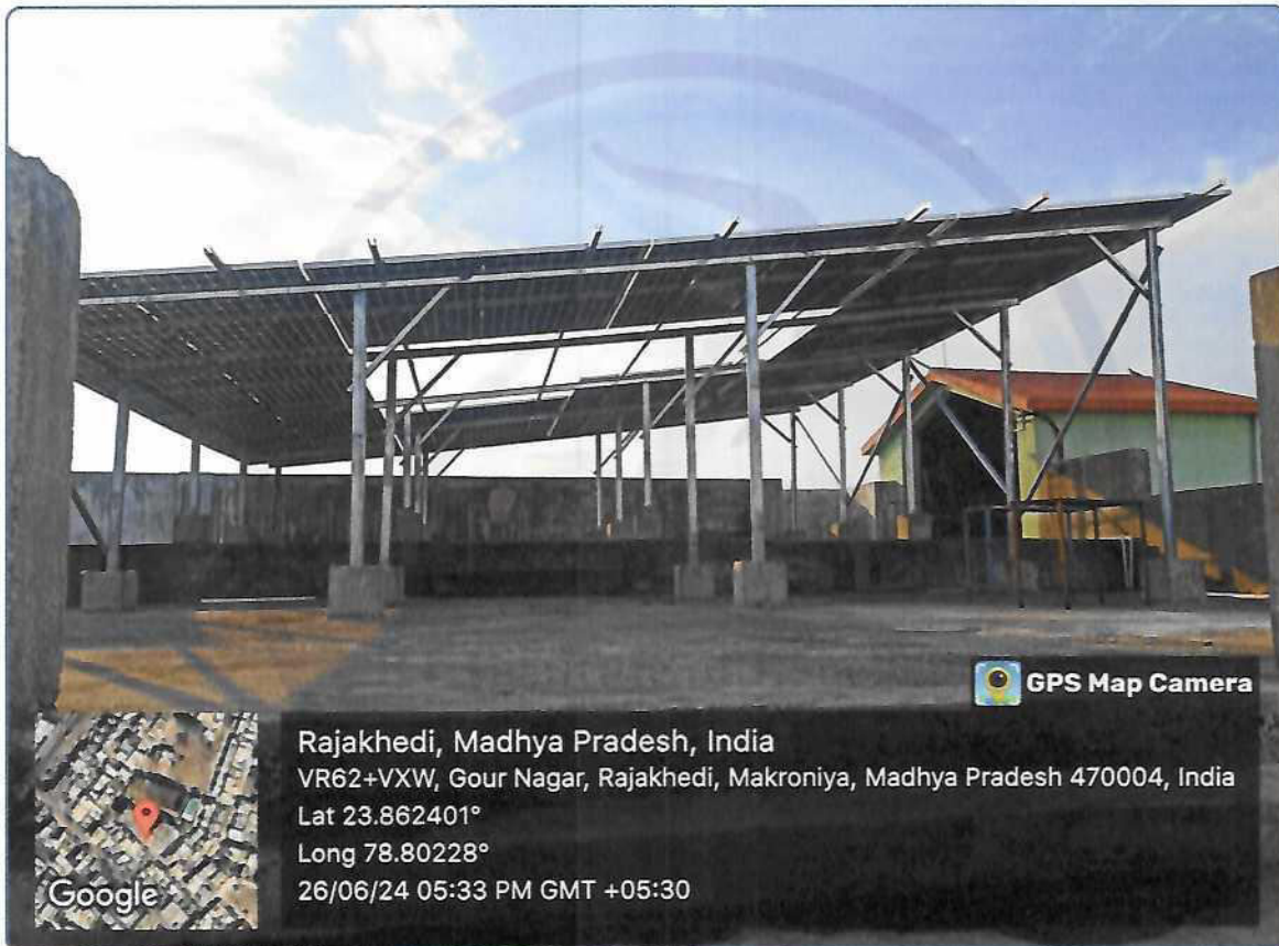
Solar System in BTIE Campus
